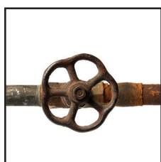
Leaking valves and fittings
